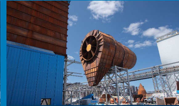
Axial Cyclone installation on Baghouse
