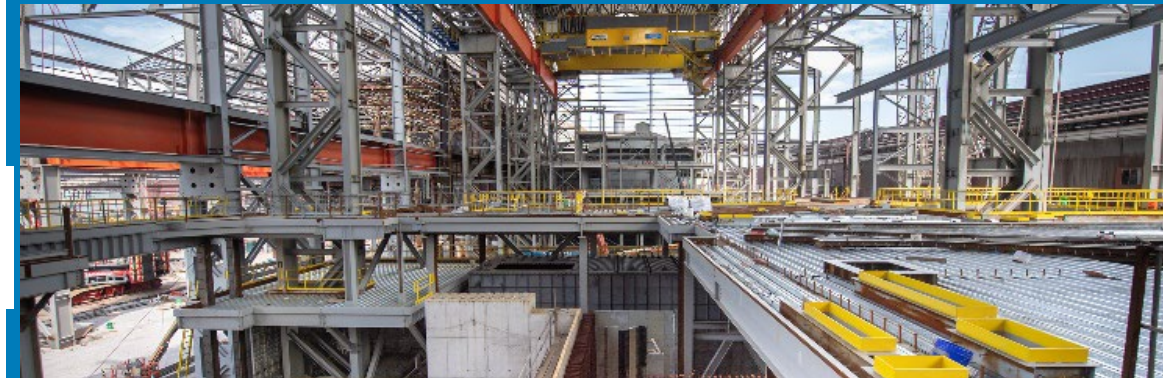
Inside view of the operating floor
